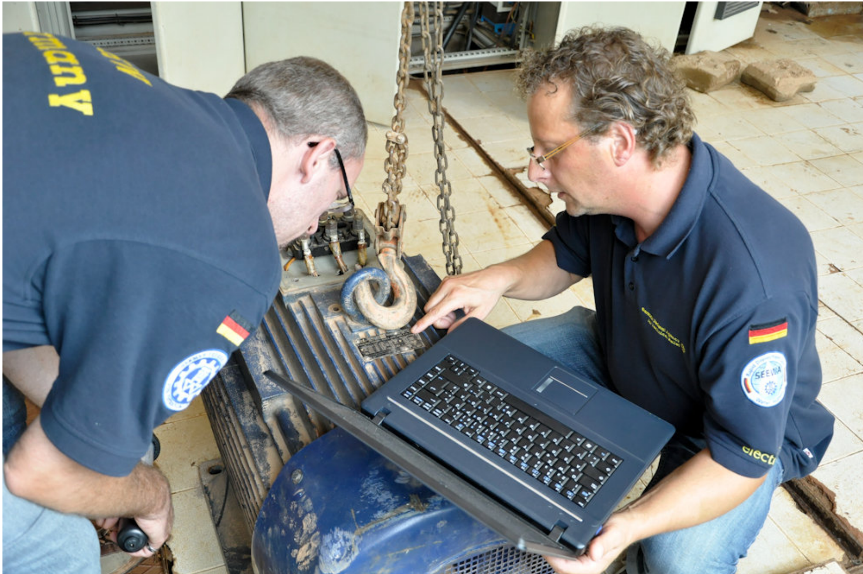
Investigation of faults to prepare the exchange of several destroyed motor pumps (produced in Germany).
